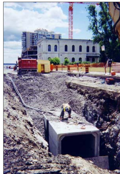
Construction of underground storage as part of sewer reconstruction along Clarence Street, in 1999.
