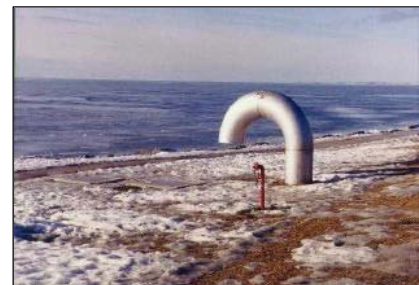
The air vent is the only visible sign of the large overflow tank at Richardson Beach
