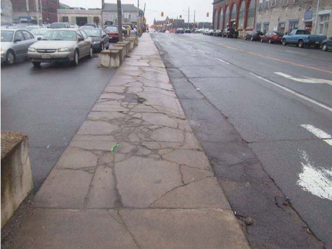
Photo 2: Cracked and Broken Sidewalks Compromise an Accessible Route on Queen Street between King and Ontario Streets
